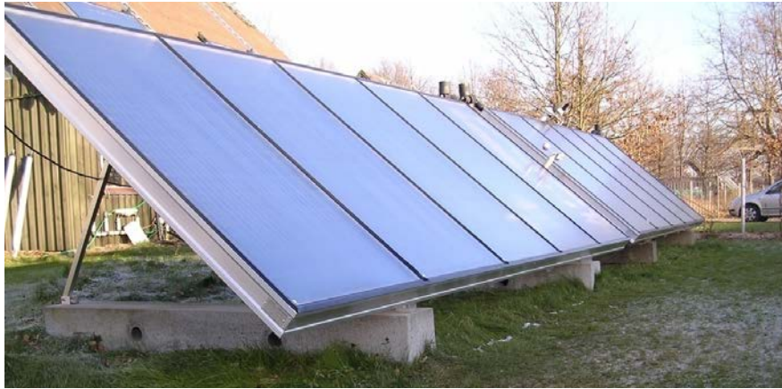
Fig. 6 Photograph of solar collector
